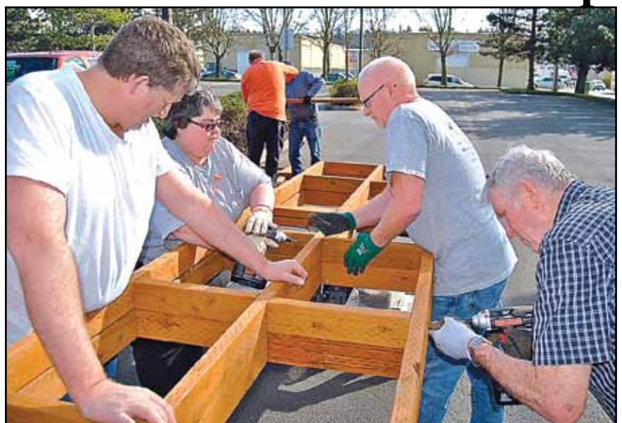
District 751 MVPs met at the Seattle Union Hall March 20 to pre-fabricate the framework for a wheelchair ramp they planned to install at the home of a Seattle woman on March 22. Building the frame in advance cuts down on final assembly time once they get on-site, said newly appointed MVP Committee Chairman Rob Curran. The group (at right) posed for a photo once they finished.
